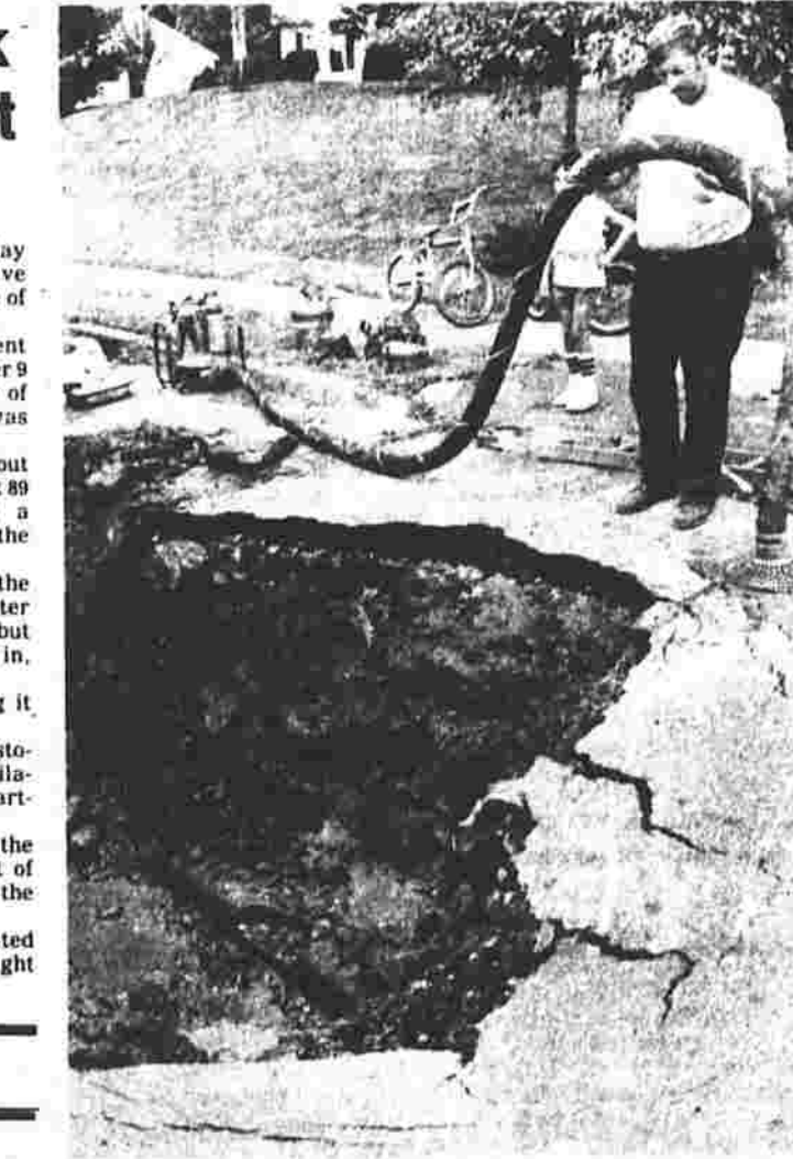
Town workers dig around a broken water main on Nutmeg Drive this morning that caused a portion of the street to collapse. The cave-in left a 15-by-8 foot hole in front of a house at 89 Nutmeg Drive.
