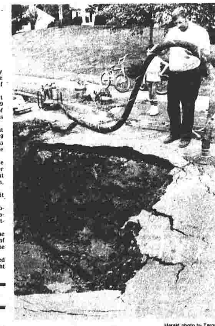
Town workers dig around a broken water main on Nutmeg Drive this morning that caused a portion of the street to collapse. The cave-in left a 15-by-8 foot hole in front of a house at 89 Nutmeg Drive.
